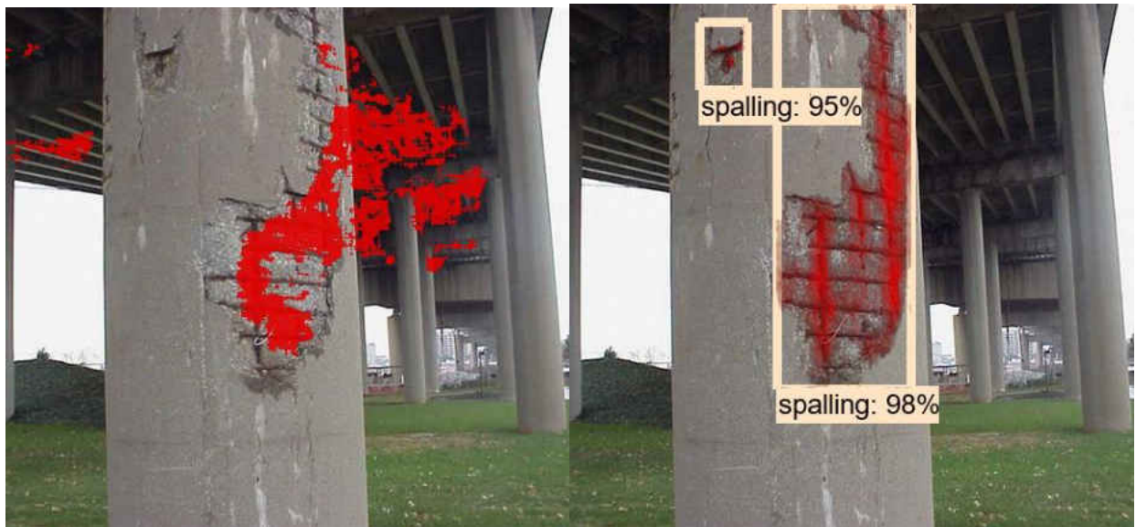
Figure 27: Effectiveness of attention guided segmentation (Left: Defect analysis resulted in some false positive results when only the segmentation model was used; Right: Misclassified pixels were readily removed when the detection pipeline created attention guidance for segmentation).
