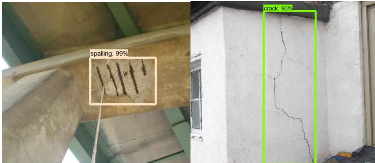
Figure 25: Damage detections on real-world images (Left: Spalling on a beam at far location, Right: Longitudinal crack located at a building wall).
