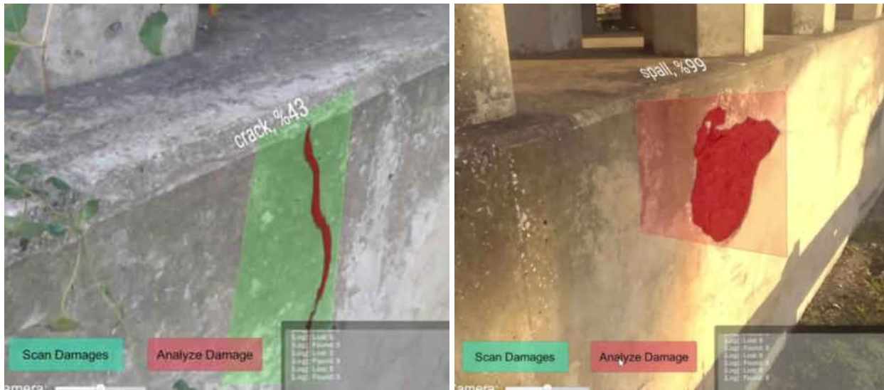
Figure 33: Real-world examples from the headset showing AI analysis results projected on the concrete defects (left: concrete crack; right: concrete spalling).
