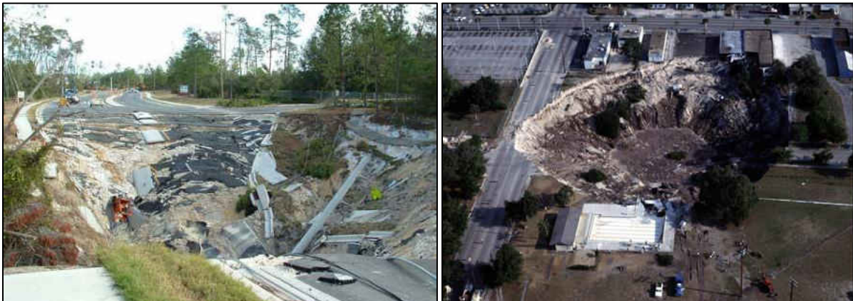
Figure 3-1: Photos of Central Florida sinkhole devastation (left: Deltona road collapse 2010; right: Winter Park 1981)
