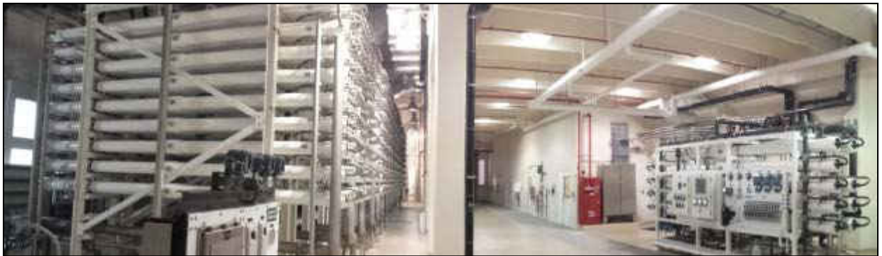
Figure 4-2: Full-scale NF trains (left) and Pilot-scale NF Unit (right) (Duranceau, 2015)
