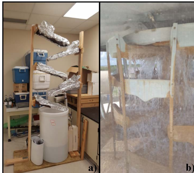
Figure 3-1: Constructed Pilot Tray Aerator (a) and Full-Scale Tray Aerator (b)
