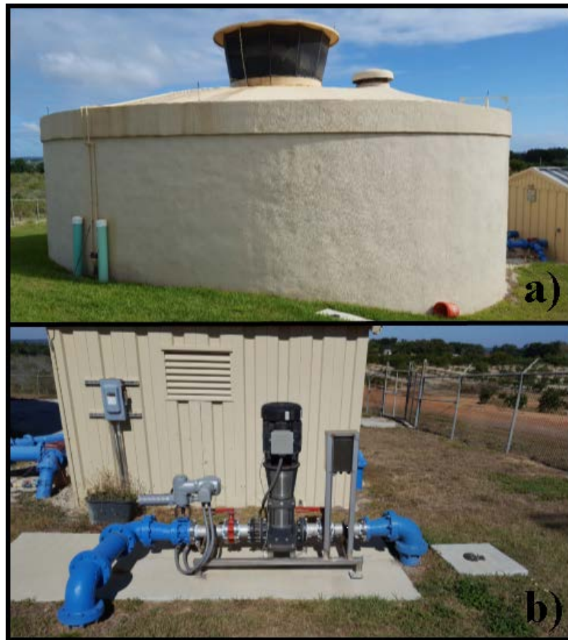
Figure 3-4: GST with Tray Aerator (a) and Recirculation Pump (b)
