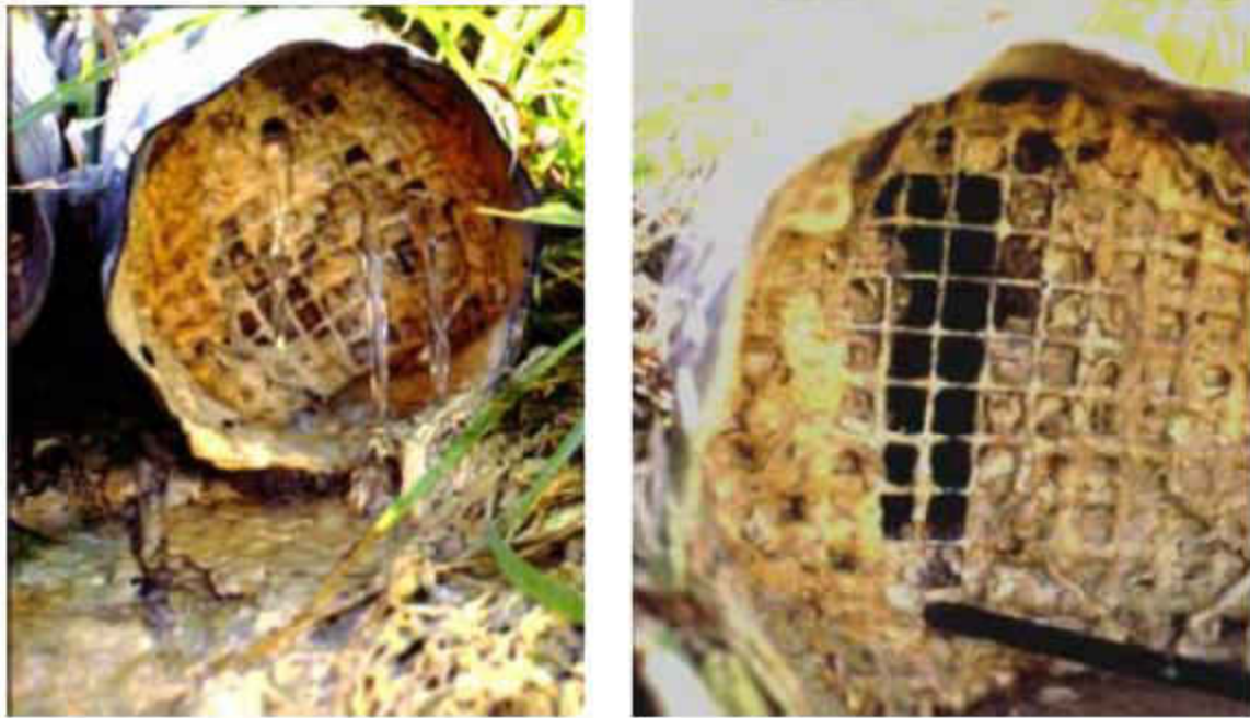
Figure 3: Clogging in drain outlet wire mesh rodent guard due to calcite precipitation (Steffes, 1999)
