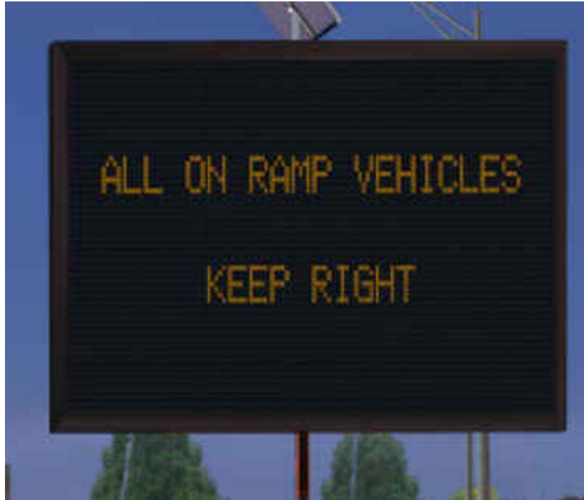
Figure 3 - 3. DMS sign that will be used for the on-ramp to keep vehicles to the right.
