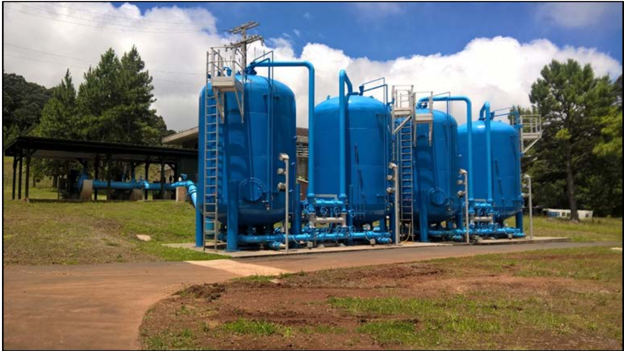
Figure 5: Pi'iholo WTP 4.0 MG GAC System
