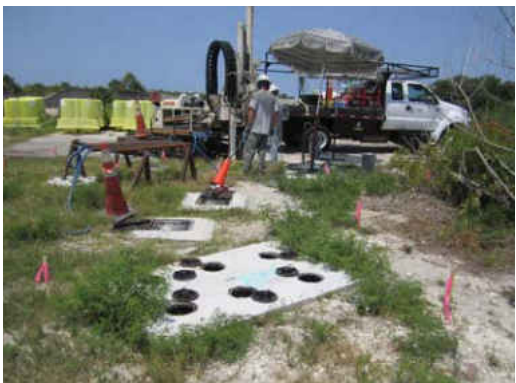
Well box locations in the injection area
