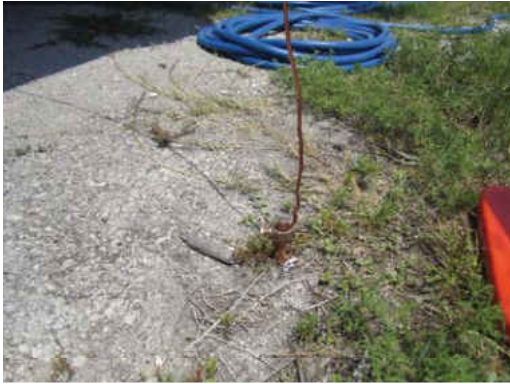
Copper spike for injection rig grounding wire
