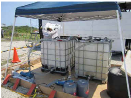
Mixing totes and transfer pumps
