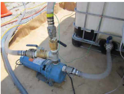
Transfer Pump bonding location
