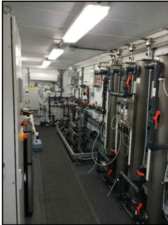
Figure A-3: Photo of interior of the ozone pilot trailer
