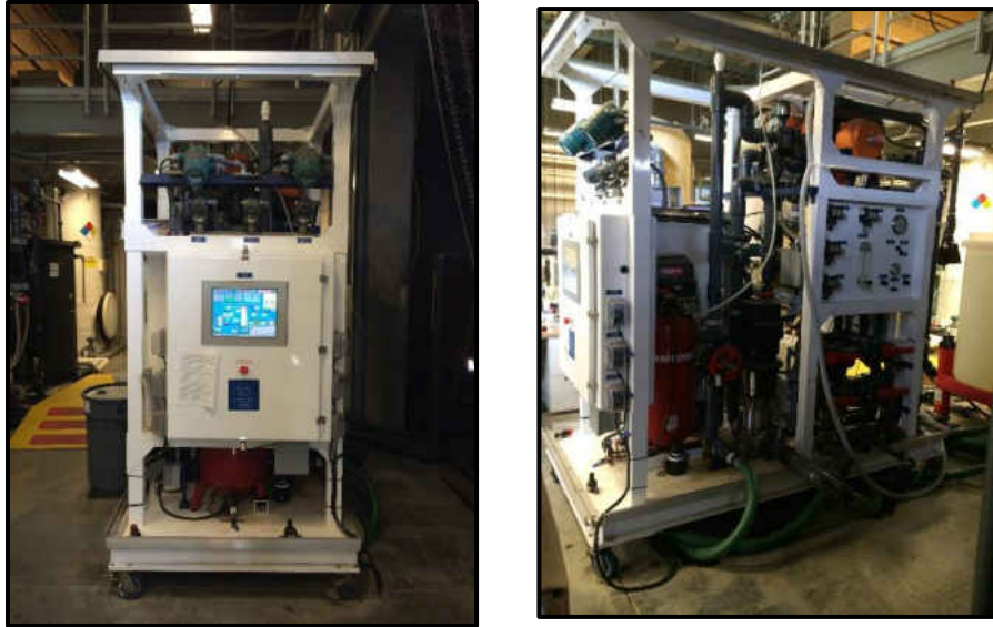
Figure A-1: Photos of the ultrafiltration pilot
