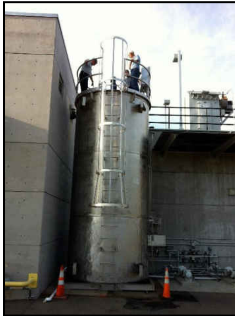
Figure A-2: Photo of the pilot-scale solid-contact clarifier
