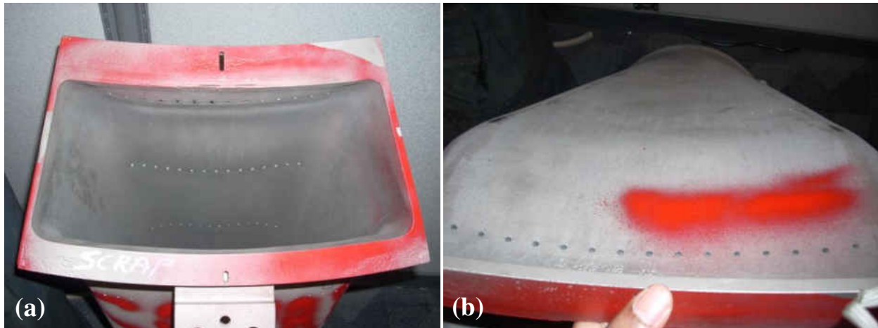
Figure 1.2 – Out of service Siemens transition piece (a) inlet connection (b) external shot of the transition path leading to outlet
