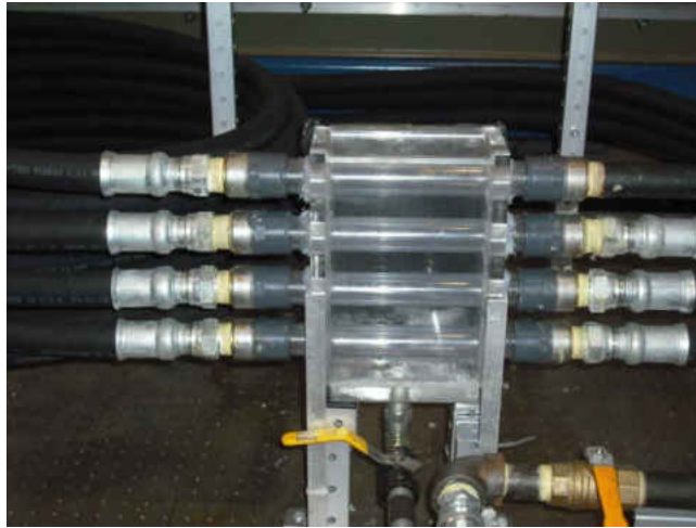
Figure 15: Flow observation box
