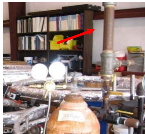
Figure 10: Scavenger injection vessel
