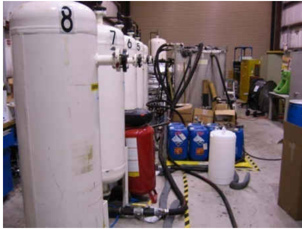
Figure 13: Scrubbing system, Tanks 6, 7, 8.
