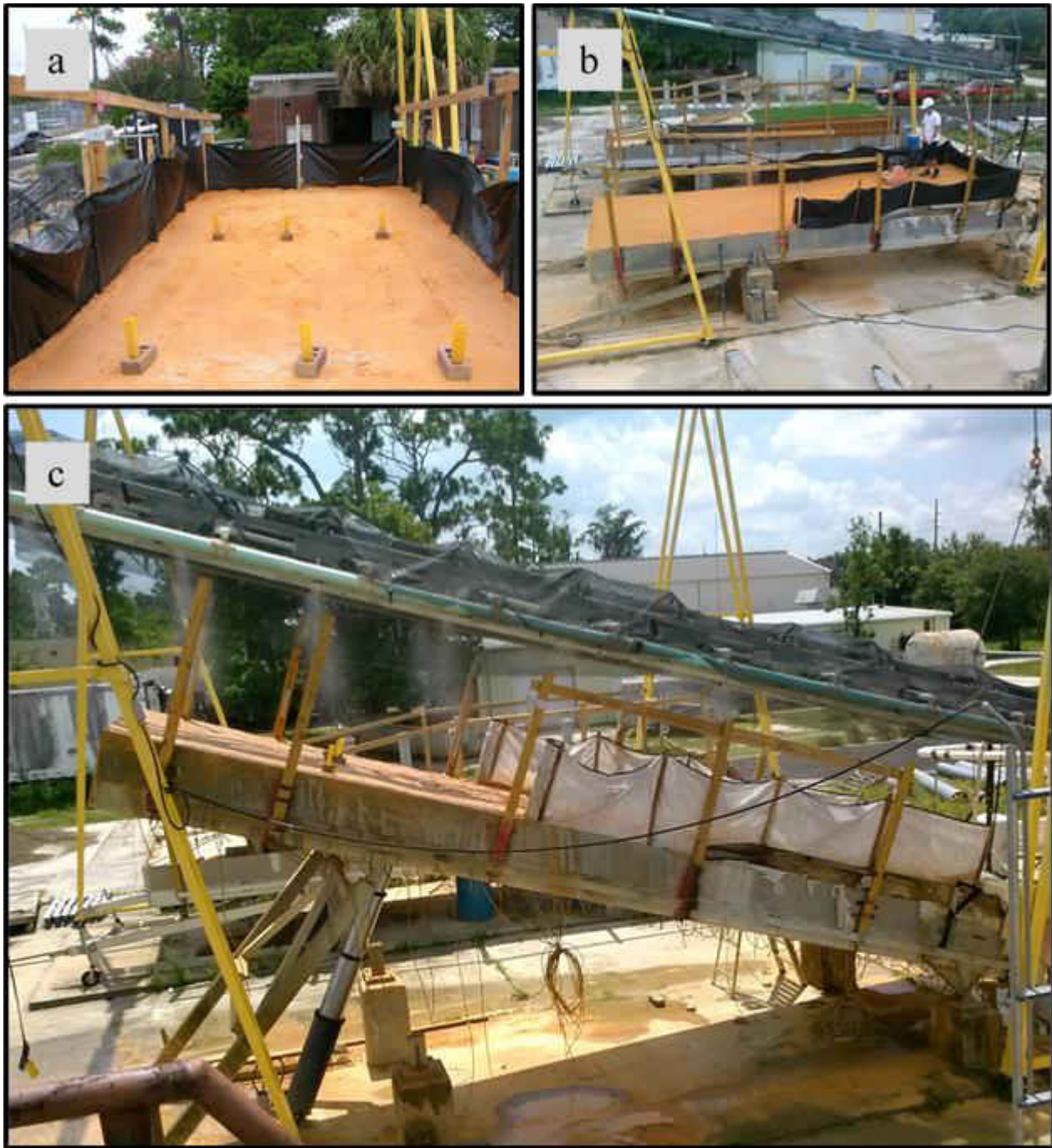
FIGURE 6 TEST BED SETUP (A) WOVEN FABRIC, RAIN GAGES, AND METER STICK INSTALLED, (B) TEST BED COMPACTION, (C) RAINFALL SIMULATOR AND TILTED TEST BED WITH NONWOVEN FABRIC INSTALLED
