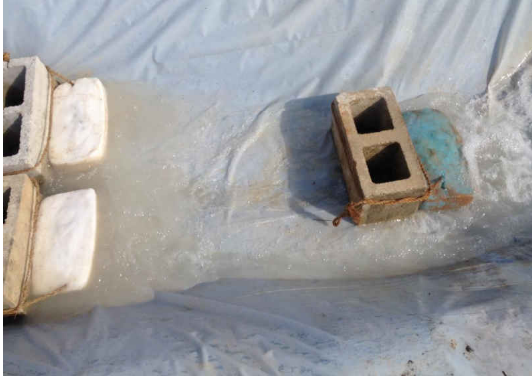
Figure 37 Crushed Limestone PAM Configuration
