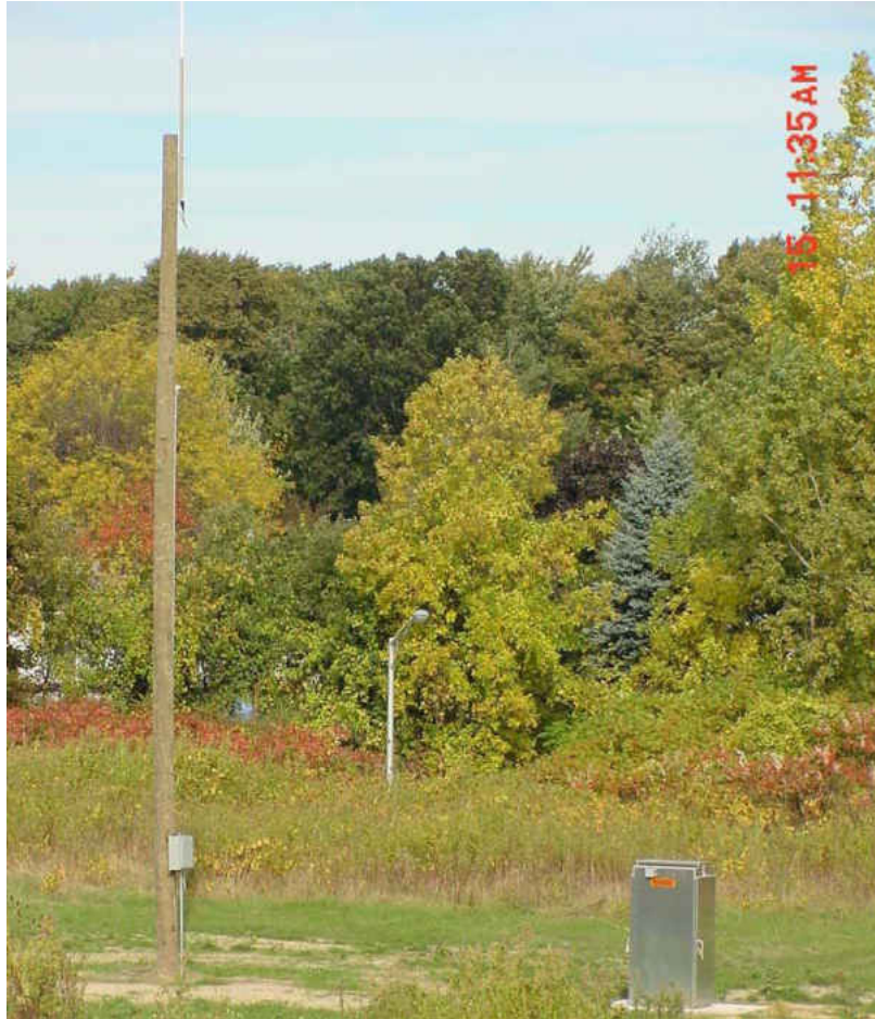
FIGURE 4 HAR STATION ALONG FREEWAY (NEUDORFF ET AL., 2003)
