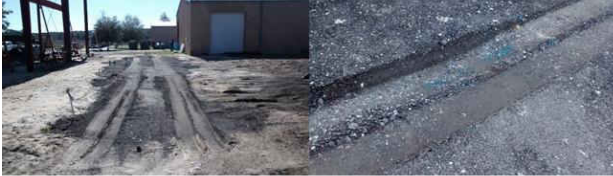
Figure 71. Deformation on milling surface
