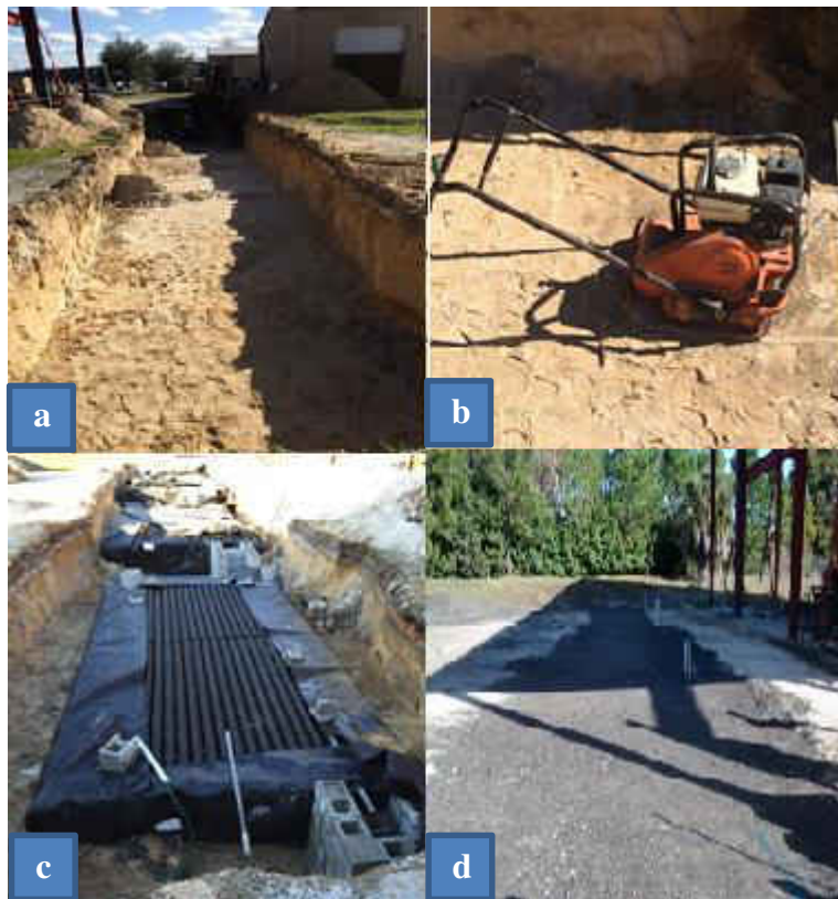
Figure 18.a. Excavated holes; b. Vibratory machine used for compaction; c. System being put into the holes; d. View of finished testing site
