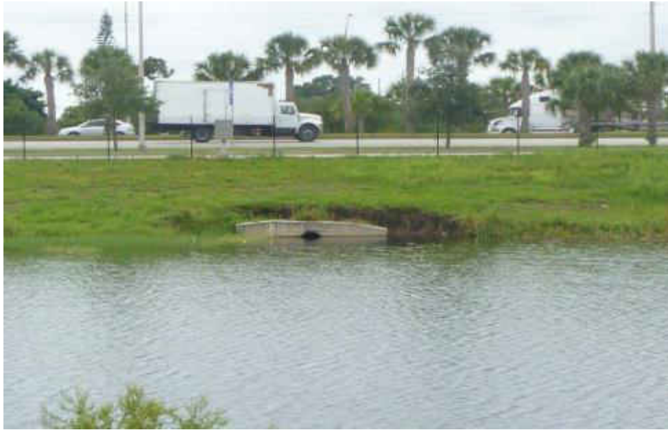
Figure 4-1 Inlet #2 displaying erosion occurring around support wall, picture taken June 2 nd , 2012.
