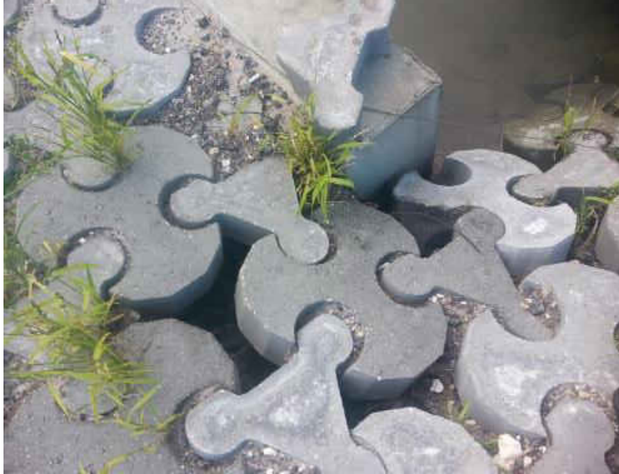
Figure 4-25 Minor erosion of fill soil between blocks occurring at the headwall edge of Inlet #2. Despite the loss of fill soil the blocks appear to retain their structural integrity.
