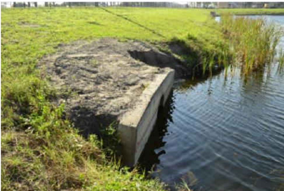
Figure 4-2 Inlet #2 displaying erosion occurring around support wall following refilling of the bank, picture taken March 1 st , 2014.
