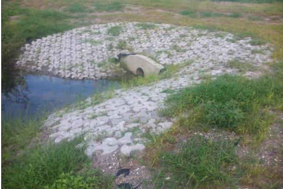
Figure 4-23 Inlet #1 two months following installation of TriLock Blocks, picture taken August 30 th , 2014.
