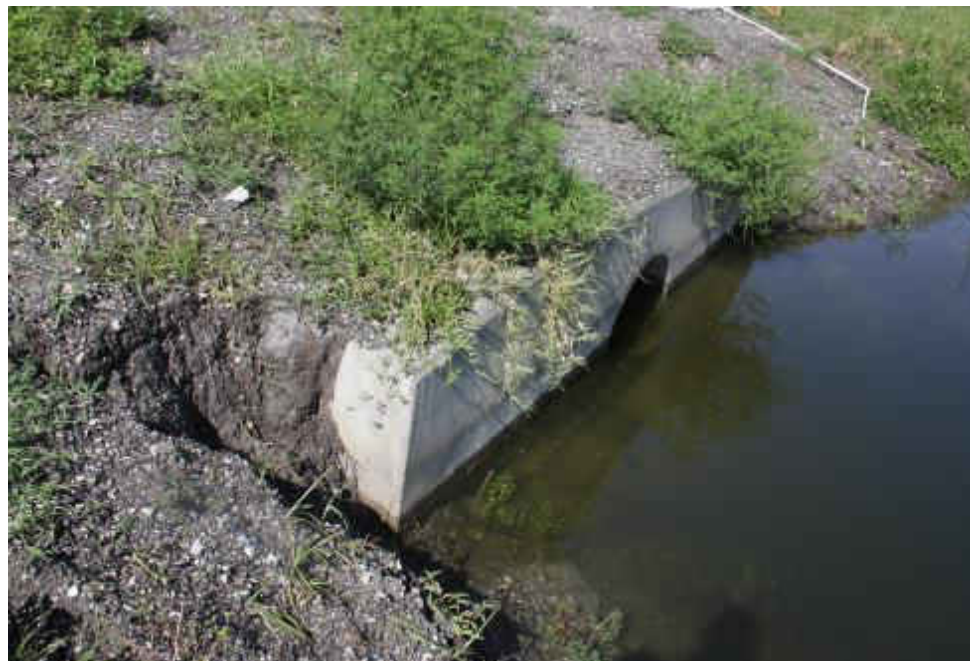
Figure 4-4 Inlet #2 erosion re-occurring around support wall three months following re-filling, picture taken March 17 th , 2014.
