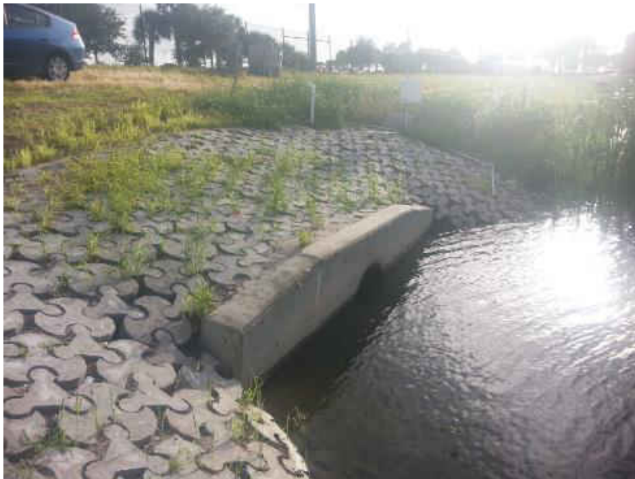
Figure 4-24 Inlet #2 two months following installation of TriLock Blocks, picture taken August 30 th , 2014.
