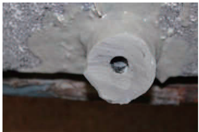
(b) Close up view of CFRP Rod slippage
