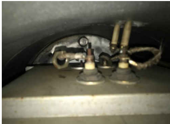
Figure 65: Wiring issue with autoclave
