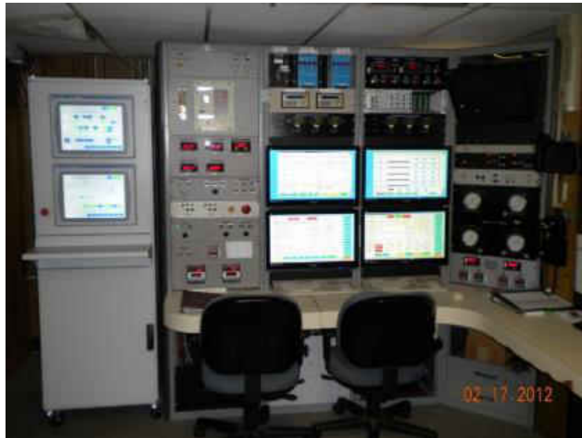
Figure A-2 LSAWT Control Room, CJES standalone console on the left. (12)
