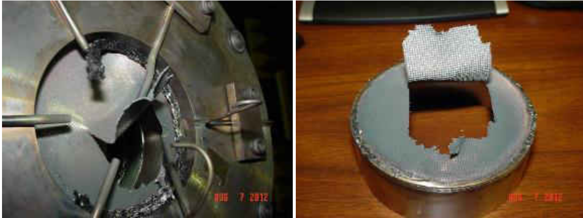
Figure 38 Second Screen Flow Conditioner Failure. (12)
