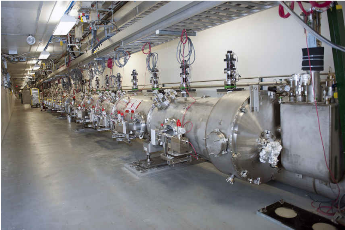
FIG. 7: New cryomodules partially installed in one of the LINACS in CEBAF. Ten cryomodules have been added to CEBAF at Jefferson Lab as part of the 12 GeV Upgrade project. Combined with the existing linear accelerators, they will double the energy of CEBAF's electron beam – from 6 GeV to 12 GeV.
