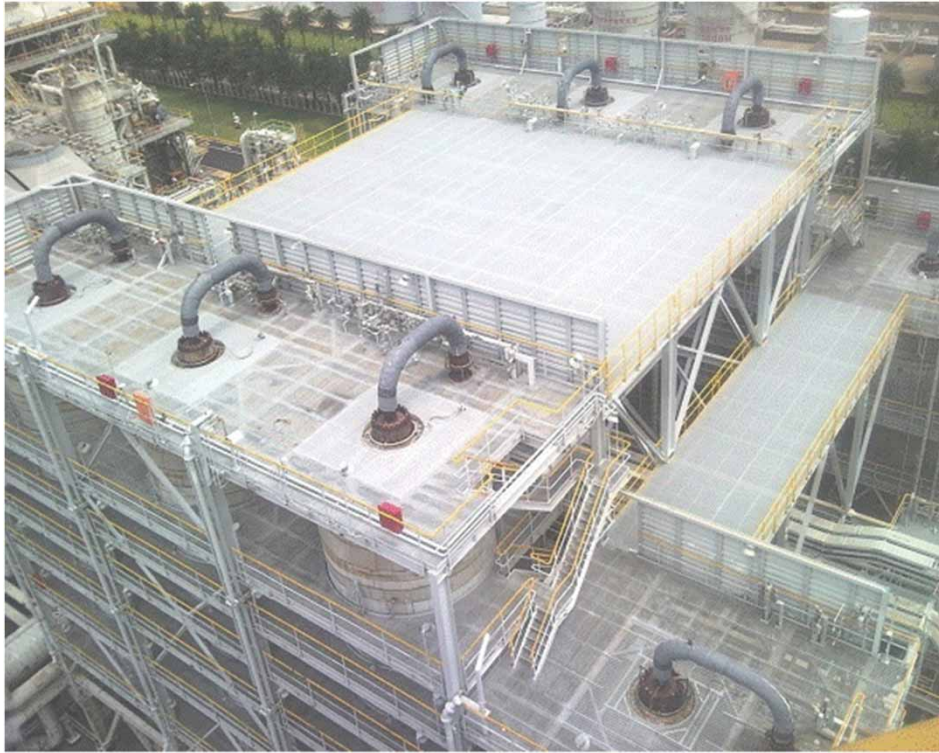
Figure 1. Residuum desulfurization (RDS) reactors and the platform.
