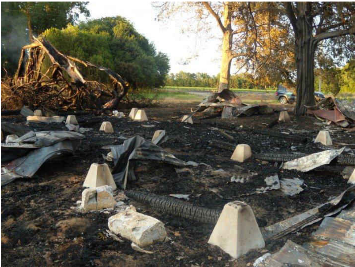
Figure 47. Photograph showing an Early 20 th Century out building constructed of beam over pilings support. Burnt 7/22/11 in Register, GA. View #1
