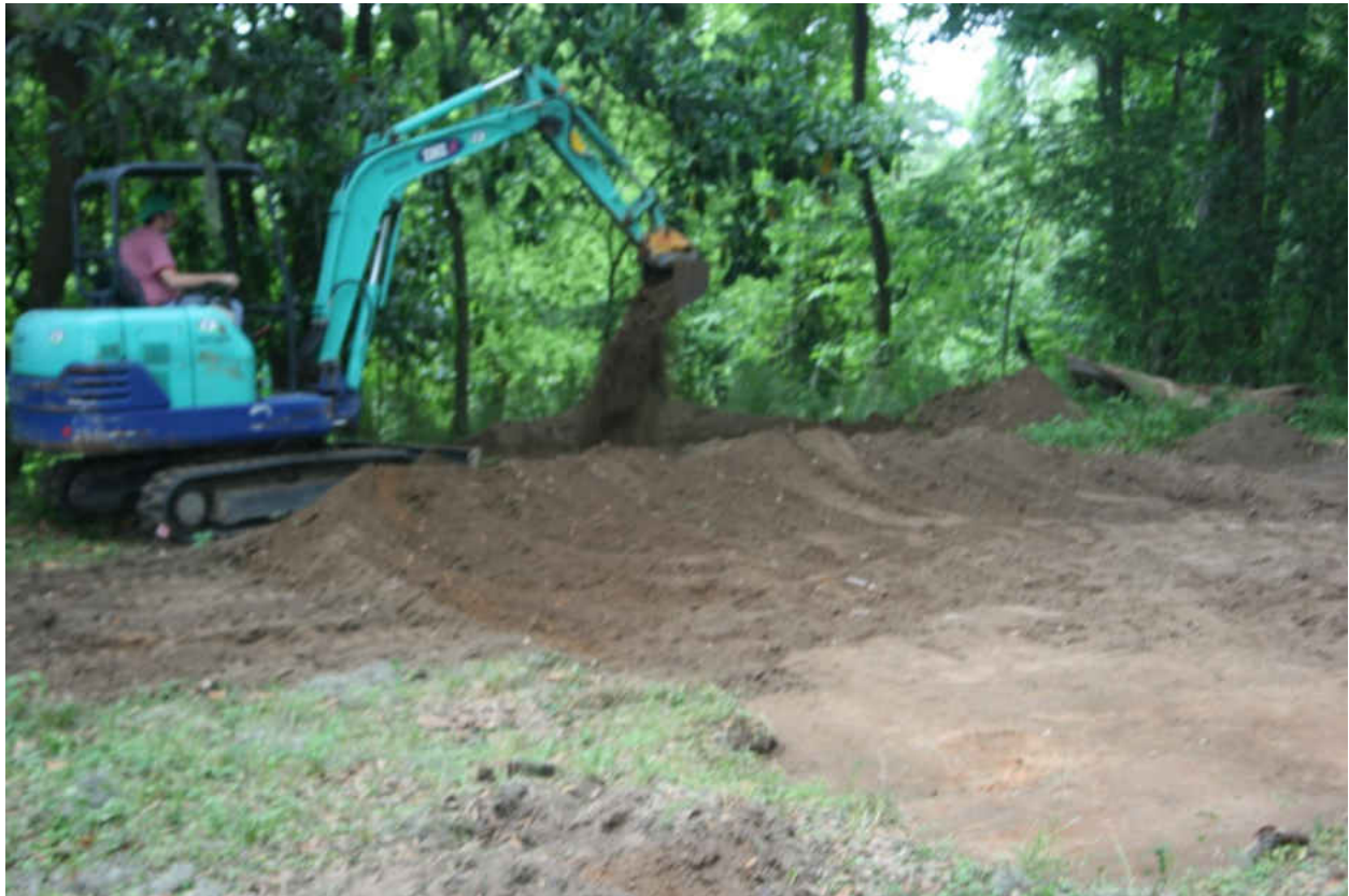
Figure 10: Mini excavator removing the plow zone from the cemetery area in May 2009.
