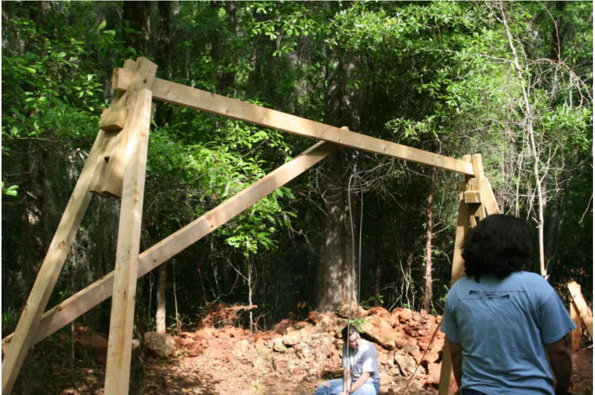
Figure 20. Picture shows the pulley system that was used to bring the buckets up from the bottom.
