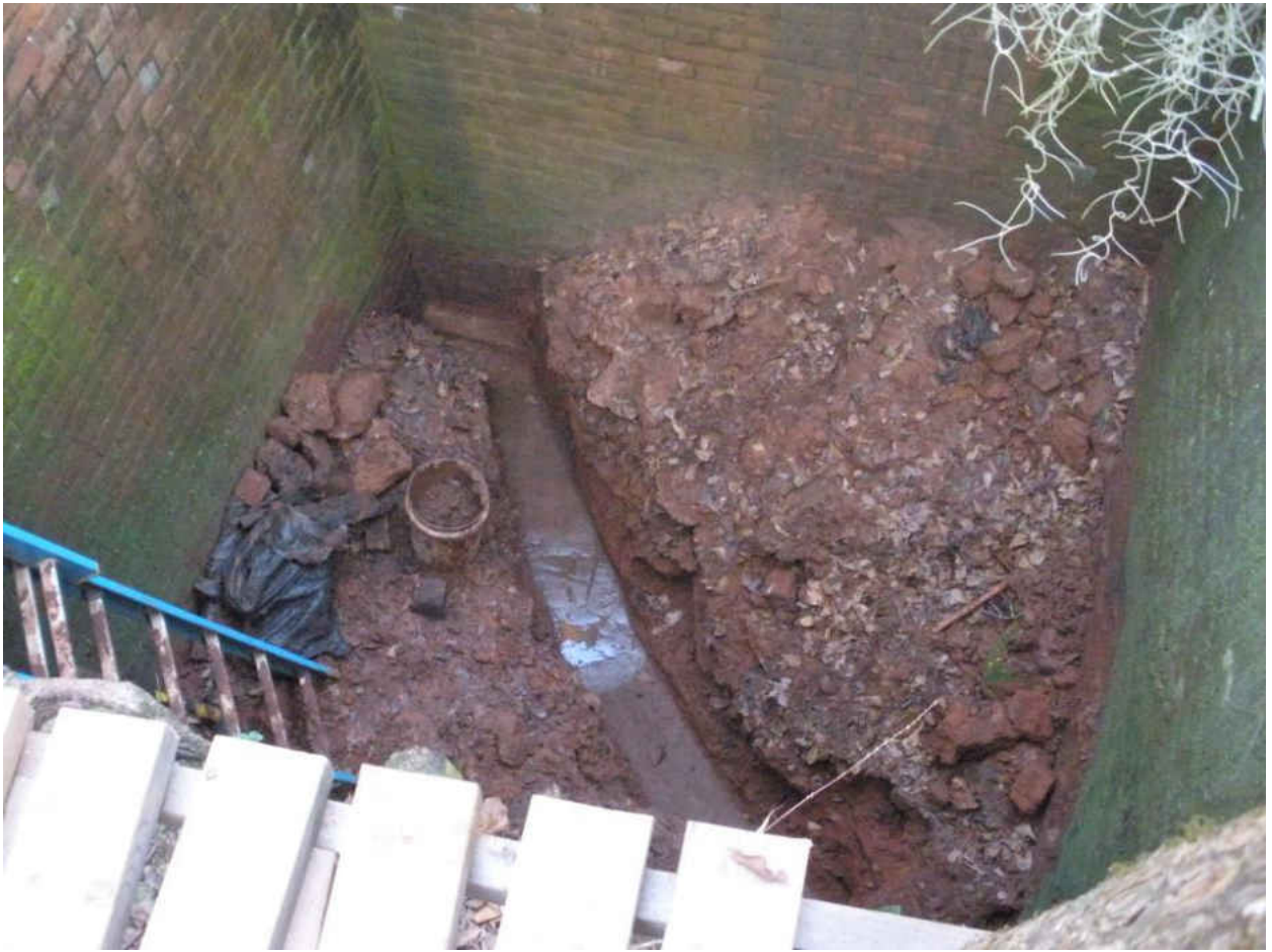
Figure 22. Picture shows the trench that was cut to reveal the brick lined floor.
