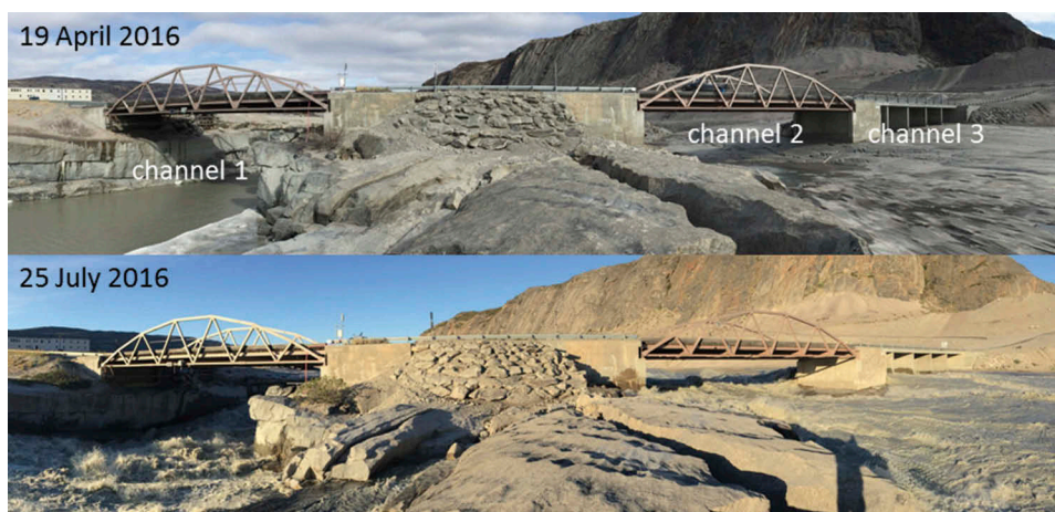
Figure 2. Gaging station at bridge crossing during low runoff (April 19, 2016) and high runoff (July 25, 2016).
