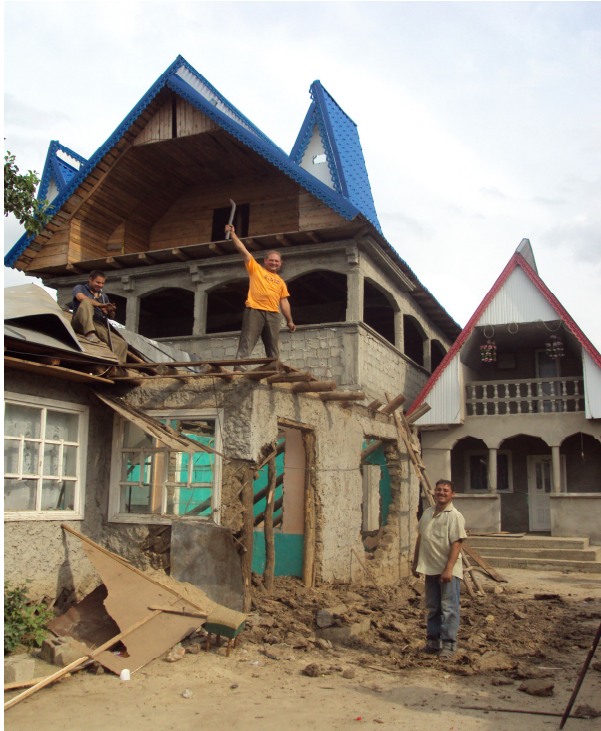
Figure 19 Caldadar man from Costesti demolishing the peasant old house in the courtyard of his new property in order to build a house for his son, Photo taken by the author 2010.
