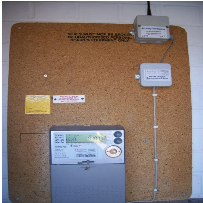
Photo 17 – Boxes which allow remote monitoring of utility meters, project from Energy School together with the company Research Machines
