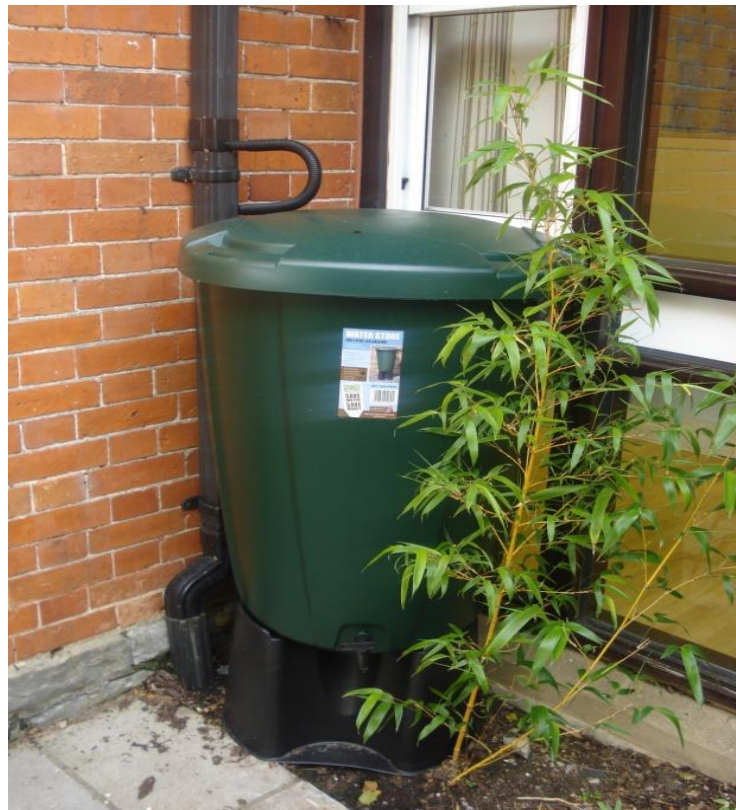
Photo 16 – Rainwater harvesting system in the grounds of Outdoor School
