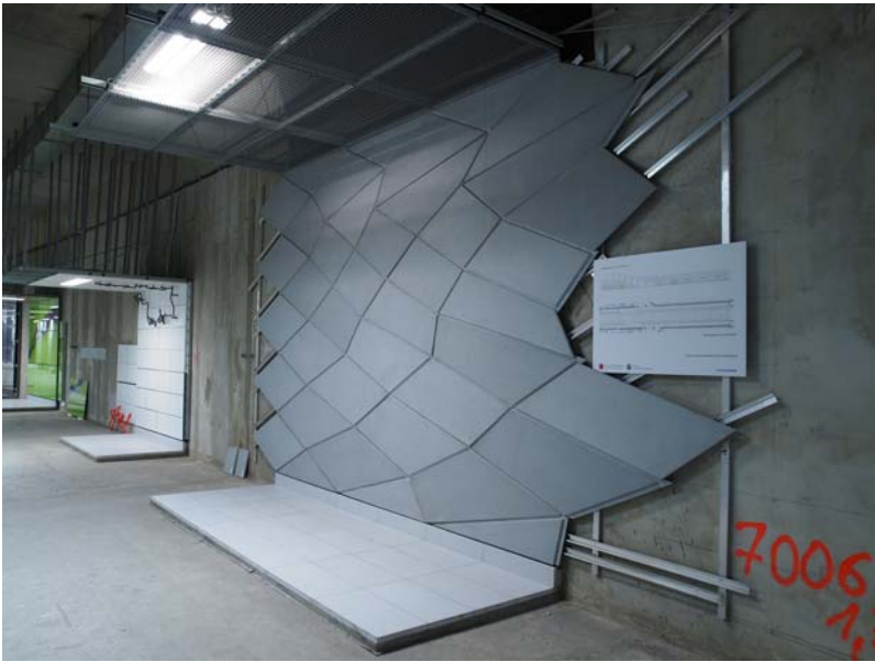
Figure 2. Developing mock-ups in advance for the new underground rapid transit line in Düsseldorf, which served to identify the best qualified project partners. © Ingo Lammert.
