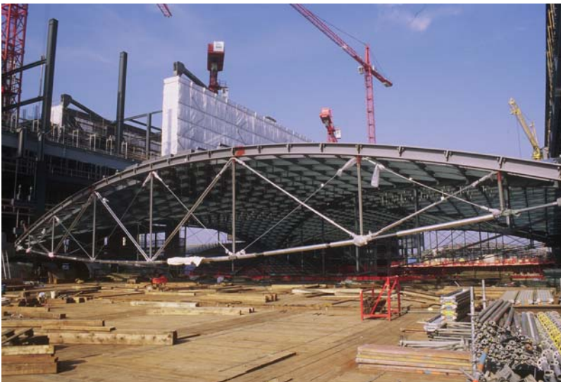
Figure 3. First time execution of vertical and overhead glazing in Germany at Berlin Central Station, which presupposed the development of new regulatory frameworks. © schlaich bergemann partner.
