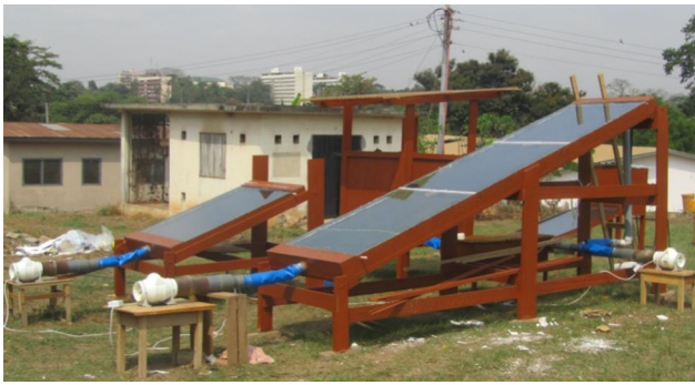
Figure 5. Collector systems: photo of construction showing the position of the fans pointed due south.
