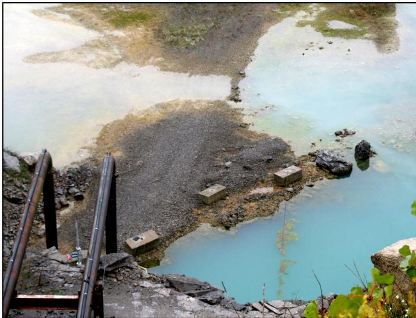
Figure 70. Photograph of pipes leading to the pump station at the southeast corner of the Hanson-Stafford Limestone Quarry (Fig. 3).
