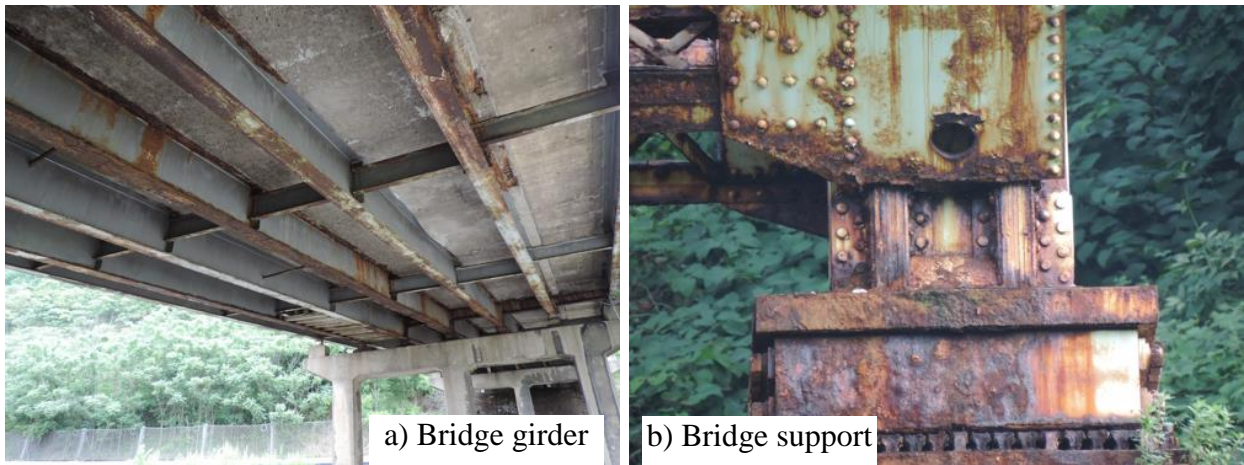
Figure 1.3: Ever-increasing corrosion in steel bridges [7].
