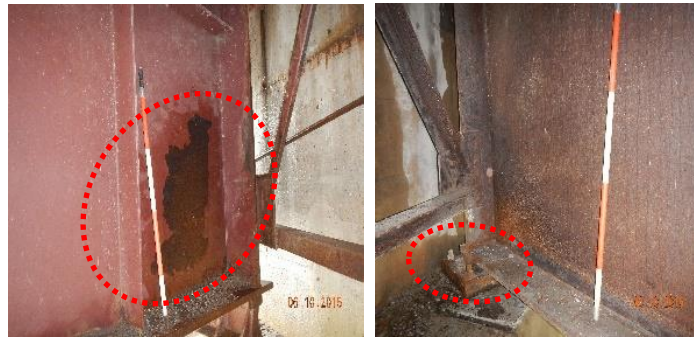
Figure 3.3: Coating failure and steel corrosion at local areas [53].
