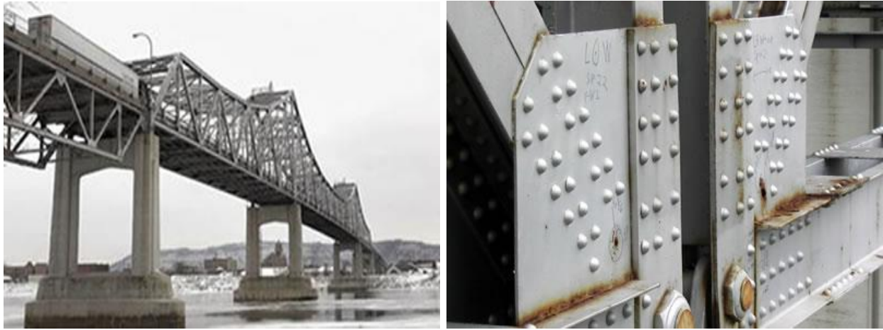
Figure 1.4: Corrosion of weldment at the gusset plates observed on the Hwy 43 bridge in Winona, MN [8].
