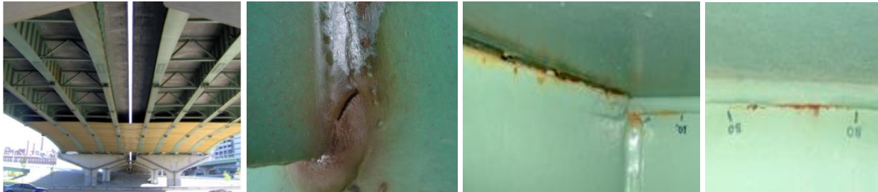
Figure 1.5: Corrosion and corrosion-induced fatigue cracks inspected at welded joints in a steel bridge [9].
