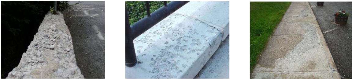
Figure 2.17. Crumbling in concrete
