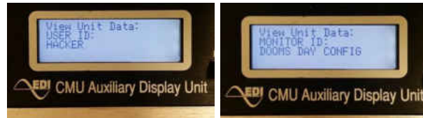
Figure 28: CMU-212 display unit showing the Datakey configuration for USER ID and MONITOR ID which was written using the home-made Arduino Datakey writer to allow for full-permissive configuration.
