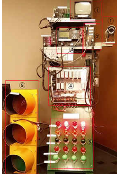
Figure 27: Traffic Signal System of TS-2 Standard. The ① is a vehicle detection and surveillance system. The ② shows the MMU-16LE while the ③ shows the Siemens Model 60 ATC. The ④ and ⑤ indicate the Load Switch relays and traffic signal bulbs, respectively.
