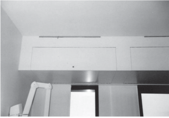
Figure 9. Air inlet-system for a hospital in a mocked-up experimental room.
