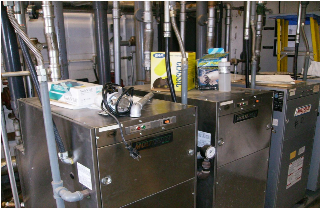
Figure 4.5 Glenburnie City gate Combustion Furnaces
