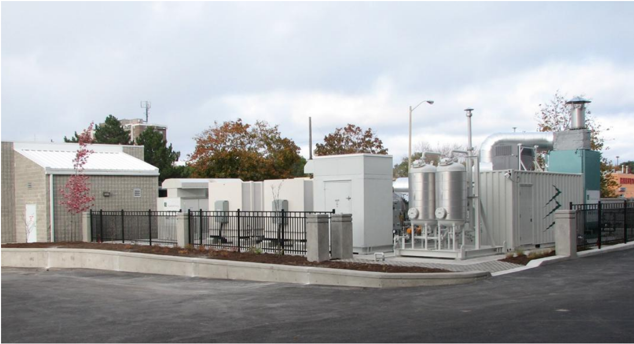
Figure 4.1 Enbridge DFC-ERG Power Plant
