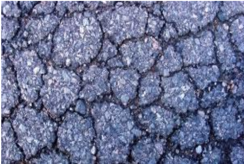
Figure 2.2: (b) Fatigue cracking (alligator cracking) [24].
