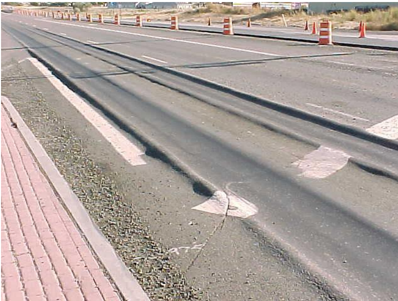
Figure 2.2: (a) Permanent pavement deformation (rutting) [22].
