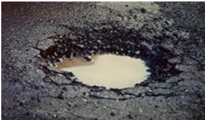
Figure 2.2: (c) Moisture damage [27].
