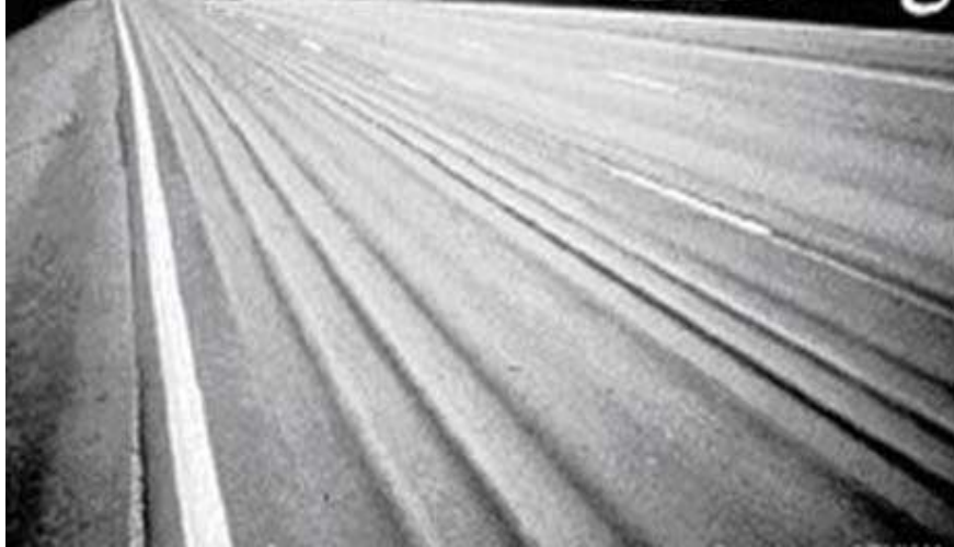
Figure 2.1 Ruts on wheel path [30].
