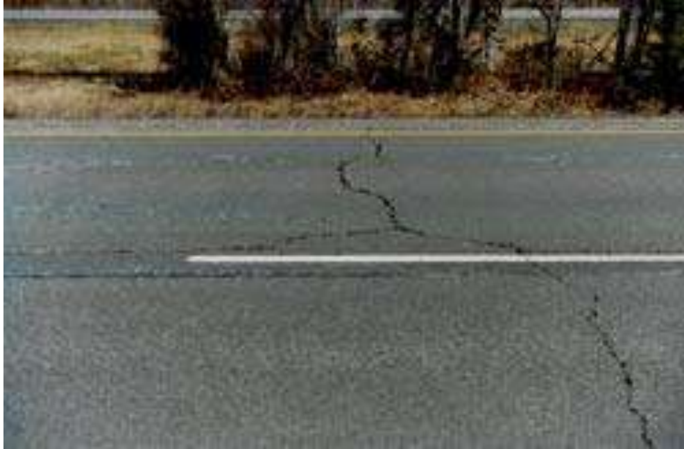
Figure 2.3: Longitudinal and transverse cracks due to thermal effects [33].
