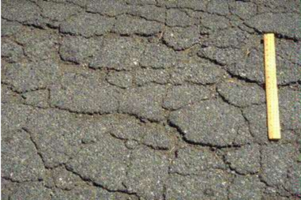
Figure 2.2: Alligator-type fatigue cracks caused by load or traffic distress [32].
