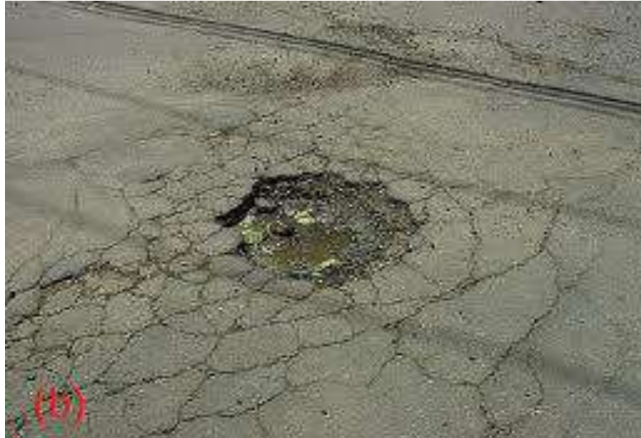
Figure: 2.4 Moisture damage [12].
