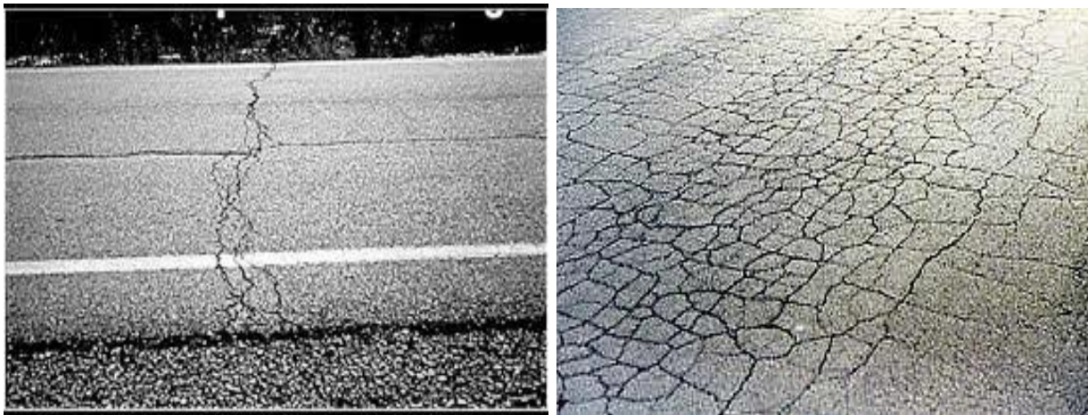
Figure 2.4: Thermal cracking of asphalt pavement [22,23].
