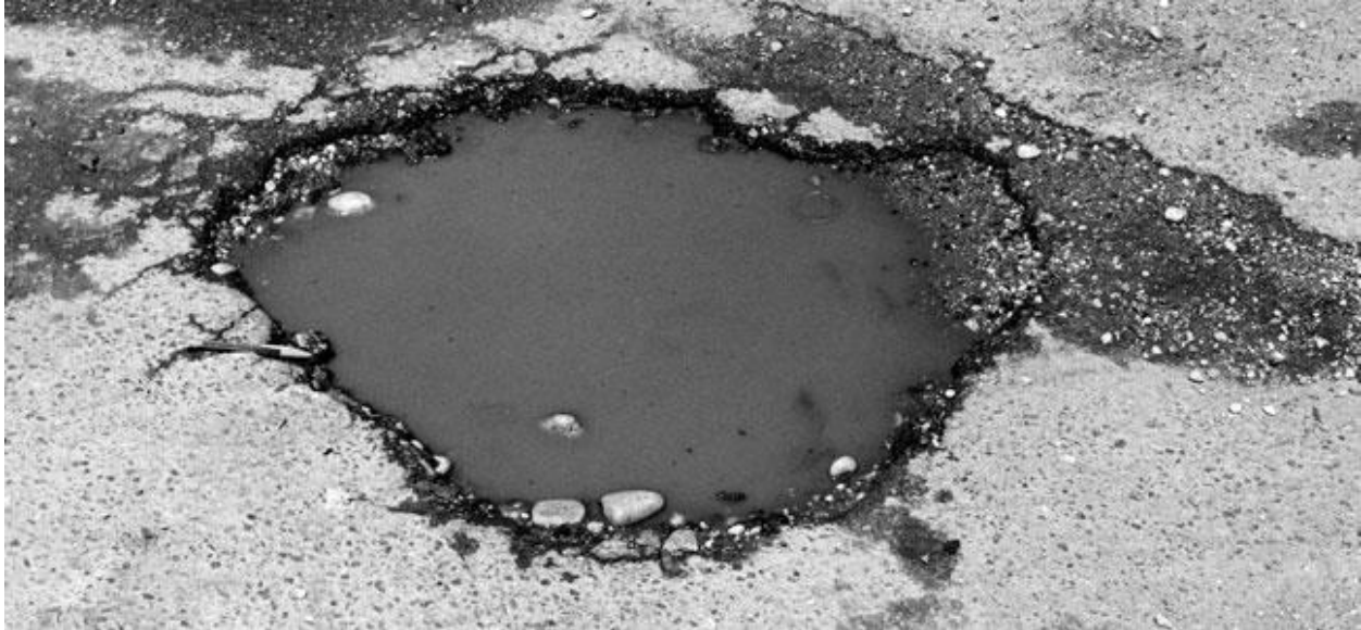
Figure 2.2: Moisture damage (stripping) [16].
