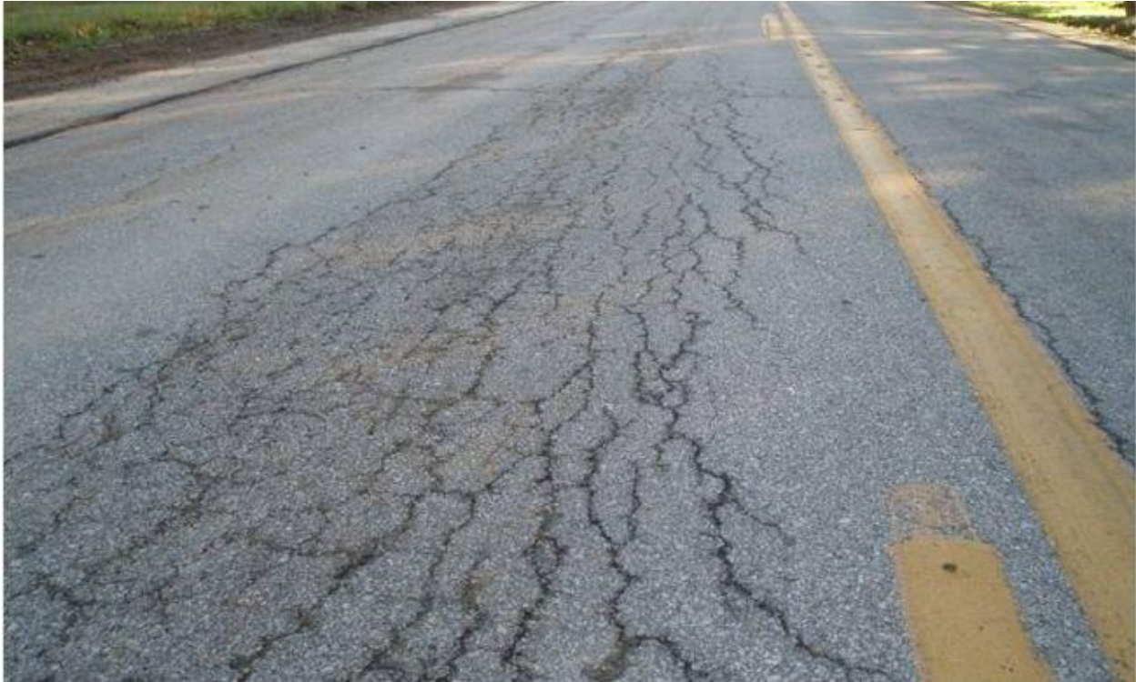
Figure 2.1: Fatigue (alligator) cracking [15].
