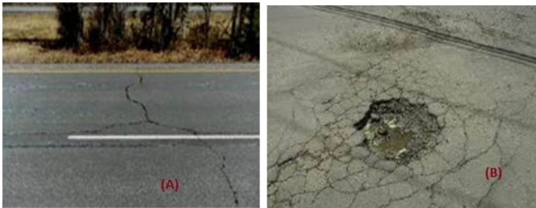
Figure 1.4: (A) Thermal cracking and (B) Moisture damage [87]
