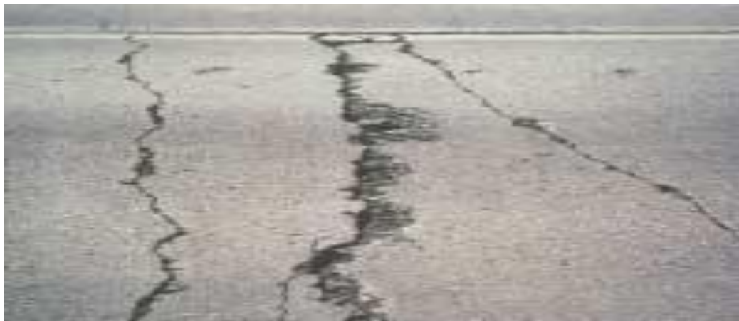
Figure-11. Transverse Cracking [50].
