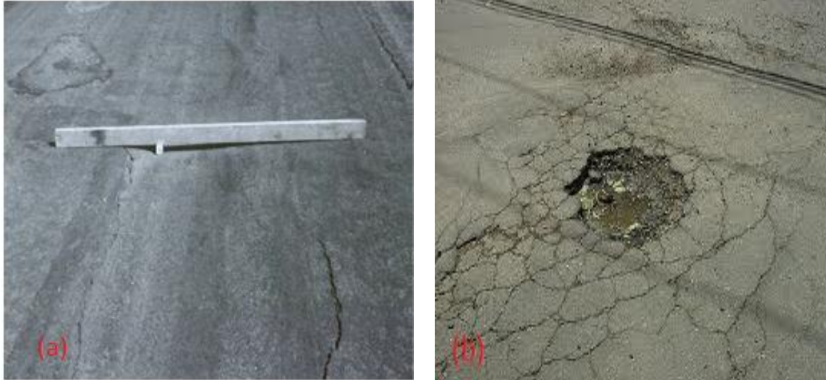
Figure 2.3: Photographs of pavements that have undergone (a) permanent deformation (rutting) and (b) moisture damage [8].
