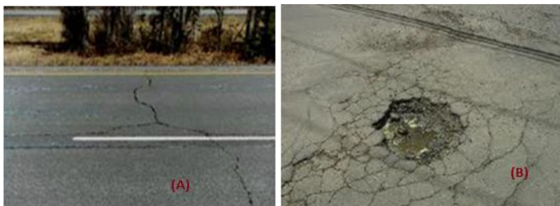
Figure 1.3: (A) Thermal cracking and (B) moisture damage.
