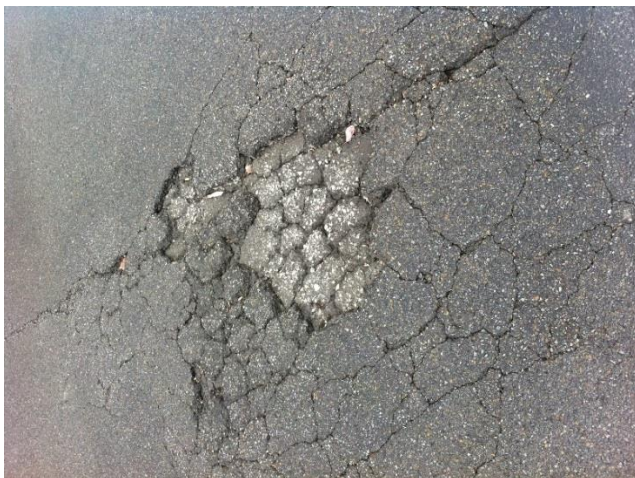
Figure 1.8 Severe fatigue distress starting to form a pothole [21].
