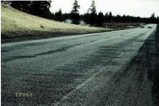
Figure 1.7 Pavement exhibiting severe ravelling [21].
