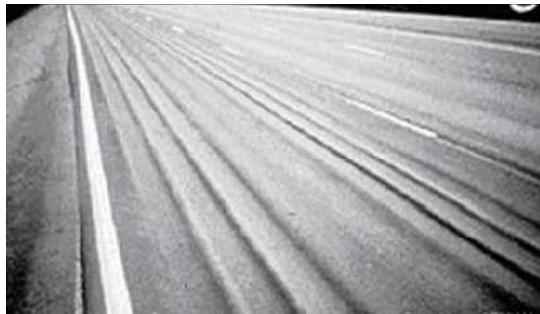
Figure 3. Severe ruts in an asphalt pavement [11].
