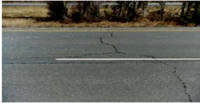
Figure 2.1 Longitudinal and transverse cracks typically due to thermal effects.
