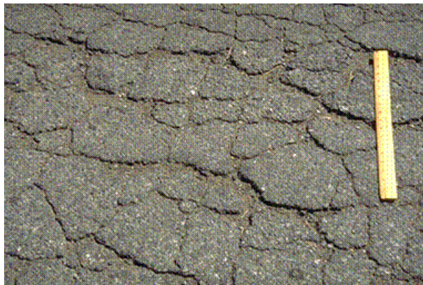
Figure 2.2 Alligator-type fatigue cracks typically due to load (traffic) distress.
