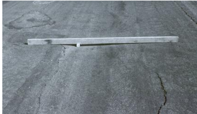
Figure 2. Measurement of rut depth on a severely damaged stretch of pavement.
