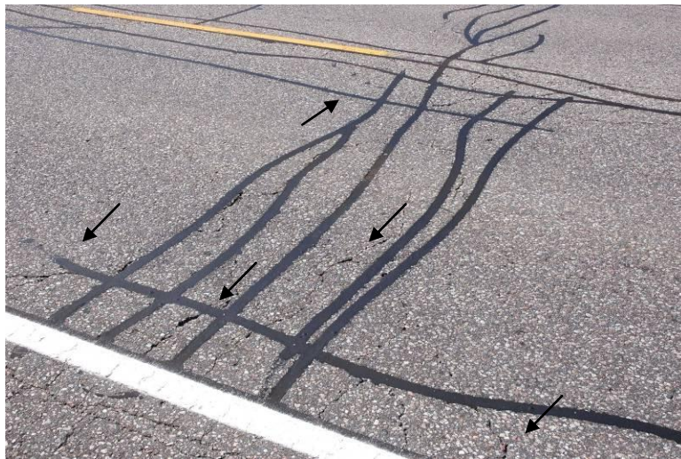
Figure 18. Typical surface condition for Highway 41 north of Kaladar. Note: Arrows indicate thermal cracks that have appeared after the original crack sealing.
