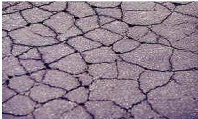
Figure 3. Area of asphalt pavement suffering from severe fatigue cracking distress.
