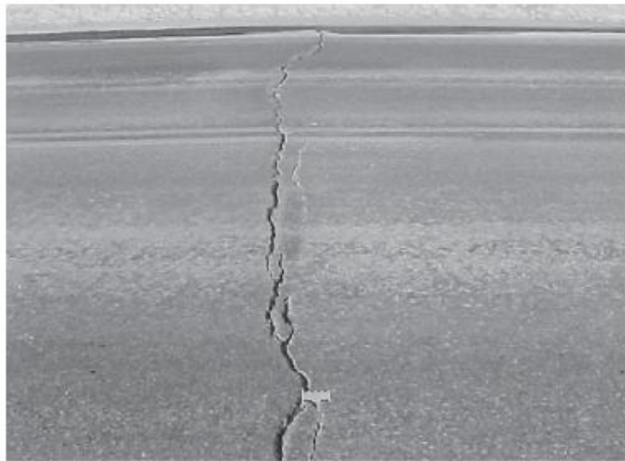
Figure 4. Typical example of a severe thermal crack in an asphalt pavement.
