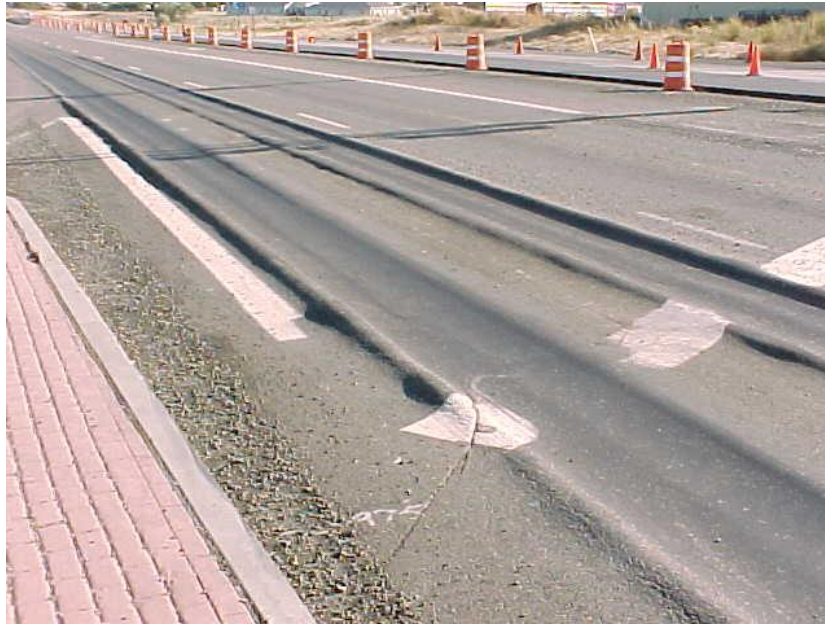
Figure 2.2: Permanent pavement deformation [35].
