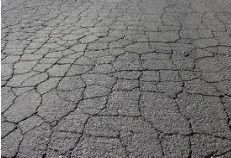
Figure 2.3: Fatigue cracking (alligator cracking) [36].
