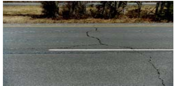
Figure 1 b. Longitudinal and transverse cracks caused by thermal effects
