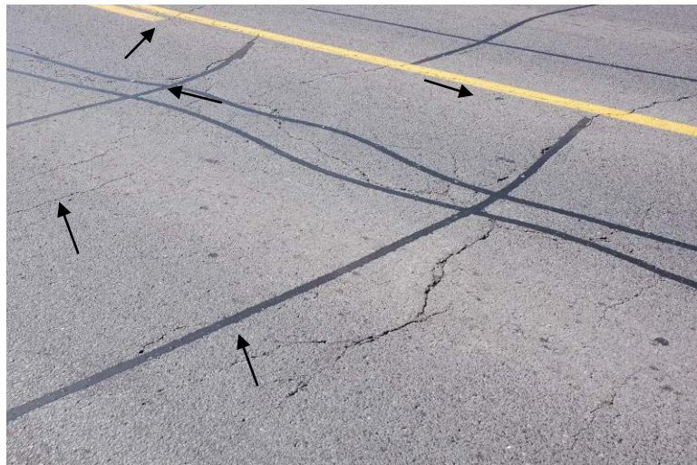
Figure 15. Surface condition of Highway 138.
