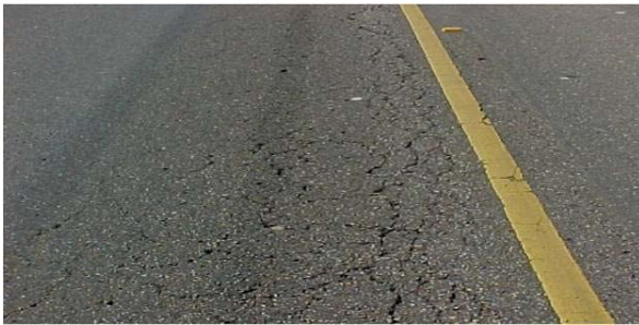
Figure 1a. Fatigue crack caused by repeated traffic loading
