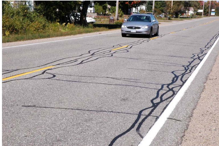
Figure 12. Surface condition for Highway 41 north of Kaladar.
