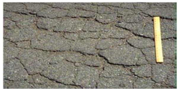
Figure 1d. Alligator-type fatigue cracks caused by load (traffic) distress
