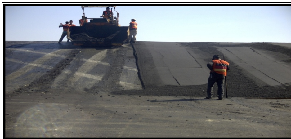
Figure 3.17: Asphalt Lining System view at Dear Al Balah Landfill (GTZ, 1996)
