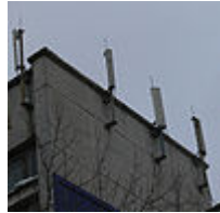
Figure(1.8) Sector antennas installed on a short mast
